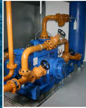
Metering system for diesel measurement
