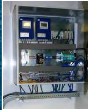
Flow Computer cabinet
